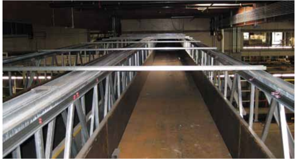
Figure 4: Double wide conveyor with lateral braces.
